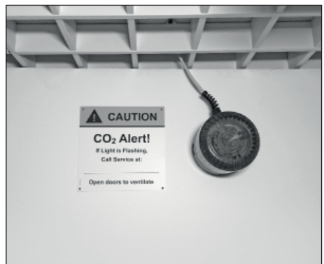
Warning lamp with sign
