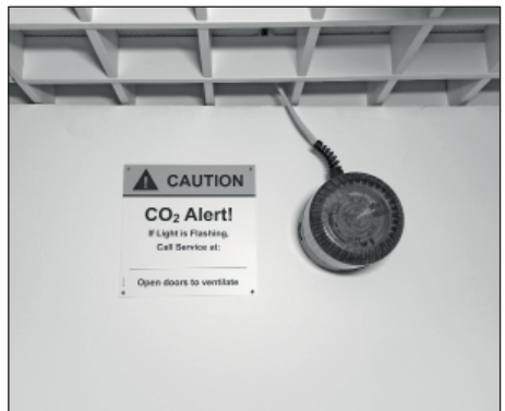
Warning lamp with sign
