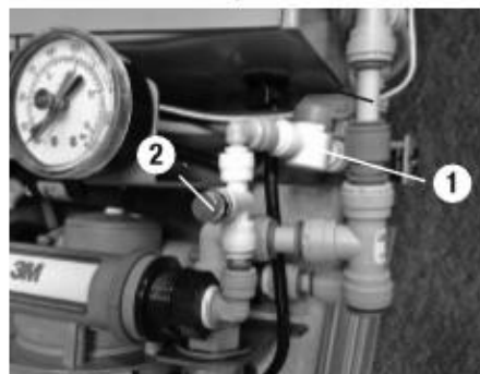
1 - blend line shutoff valve 2 - blending valve
