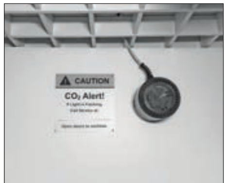
Warning lamp with sign
