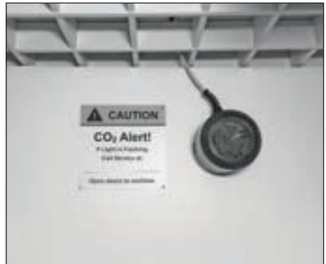
Warning lamp with sign
