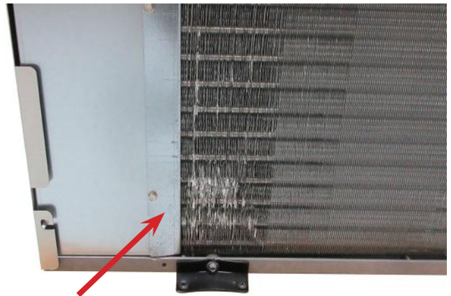
Minor fin damage close-up
